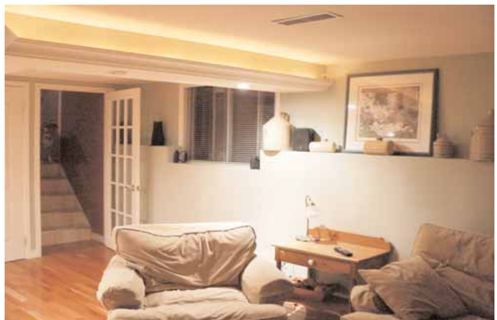
Heating plenum disguised as lighting fixture Photo by John Burrows
